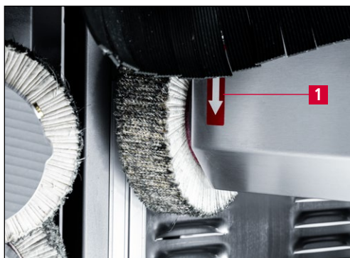
Figure 6-5 Checking rotating direction
